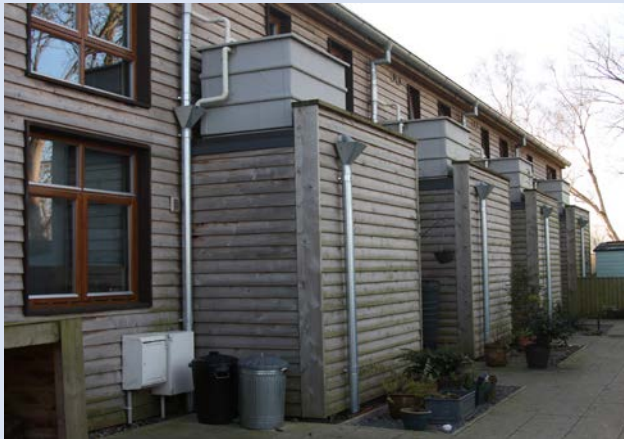
FIGURE 25: HOME RAINWATER CAPTURE SYSTEMS
